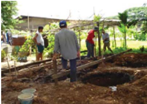
Thais and migrants in the target community build toilets with equipment and materials supported by the MHP.
